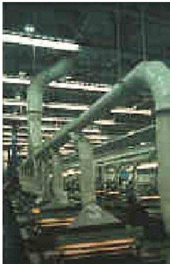
Figure 3-14. Stationary hood in an industrial process
