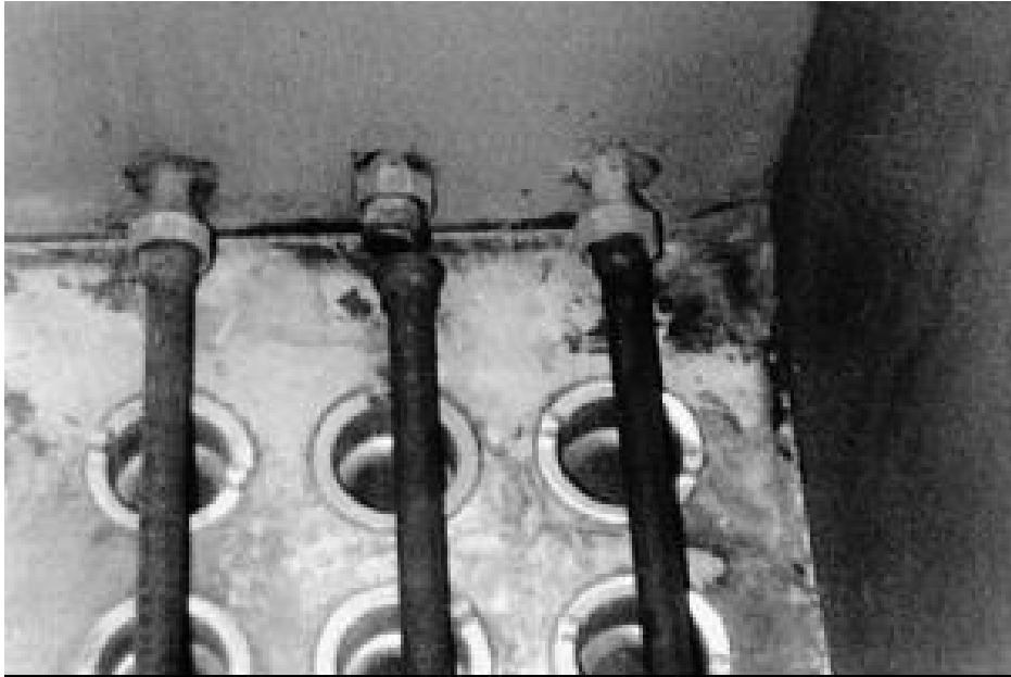
Figure 4-4. Damage to the compressed air delivery tube position relative to the bag inlet
