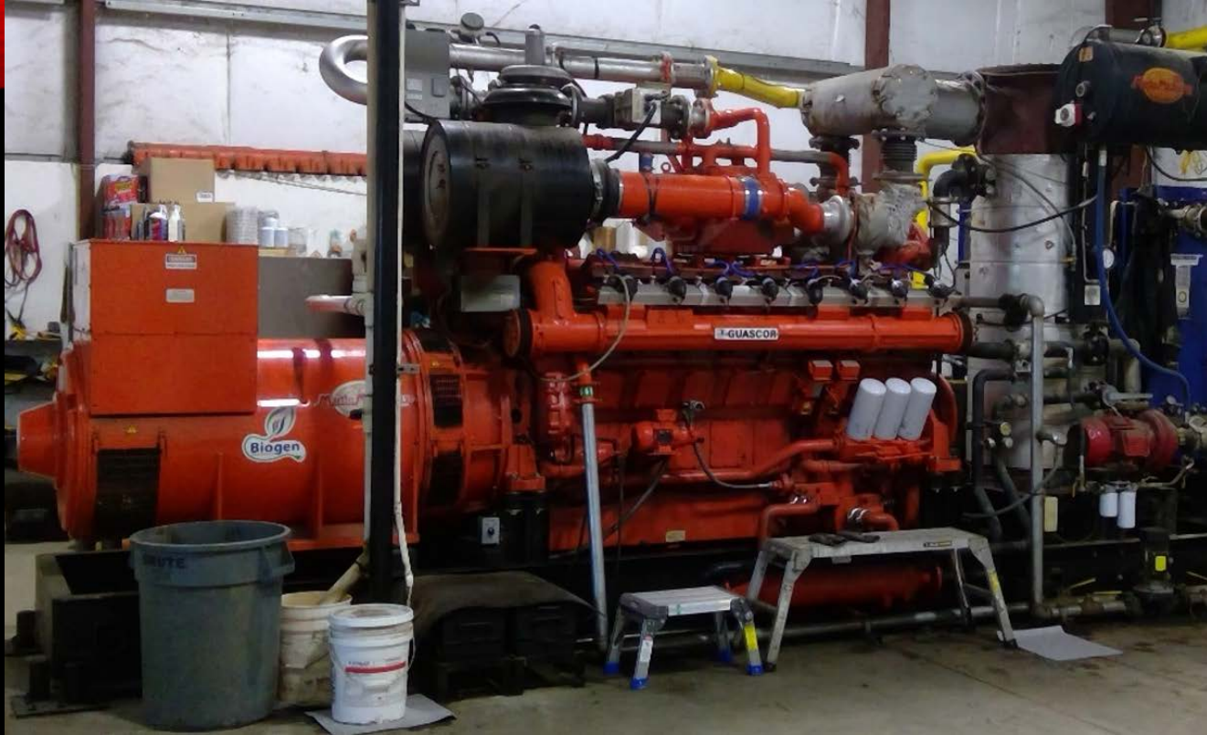
1,057 hp engine with 750 kWh generator
