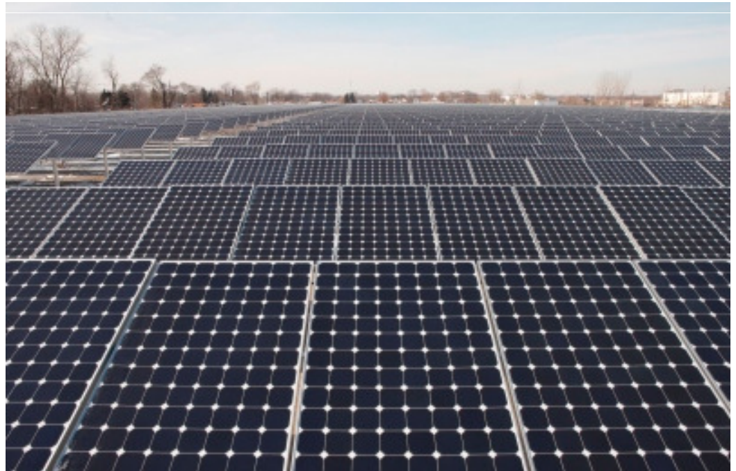
Exelon Solar Panels Chicago Southwest side Pullman neighborhood
