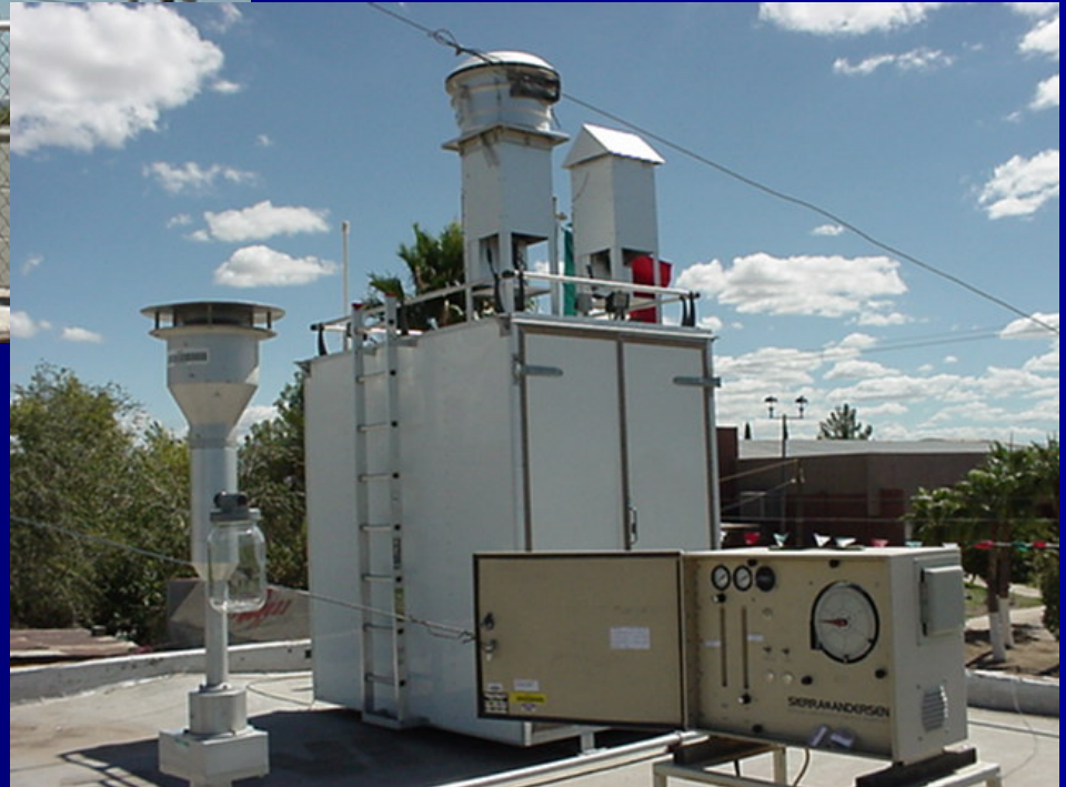
Agua Prieta, Sonora (co-located with electric power plant PM monitoring equipment)
